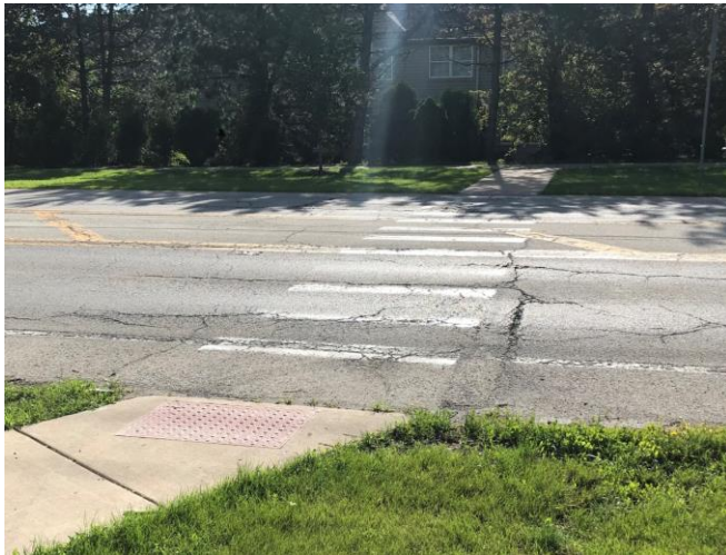
Wolf Road pavement conditions necessitate full reconstruction for better long-term performance.
